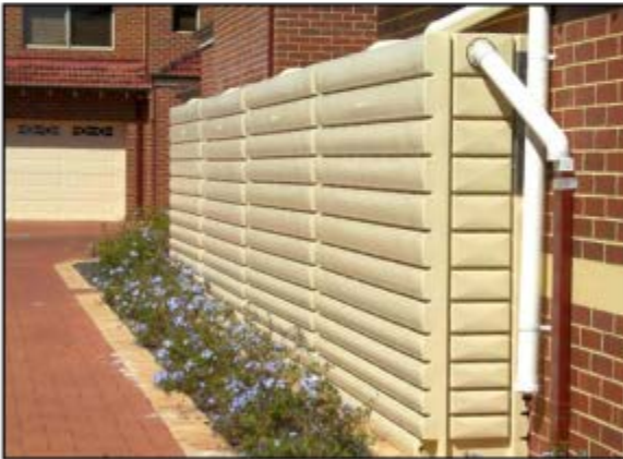
Rainwater Harvesting tanks for residential water supply at Perth, Australia 2 .
